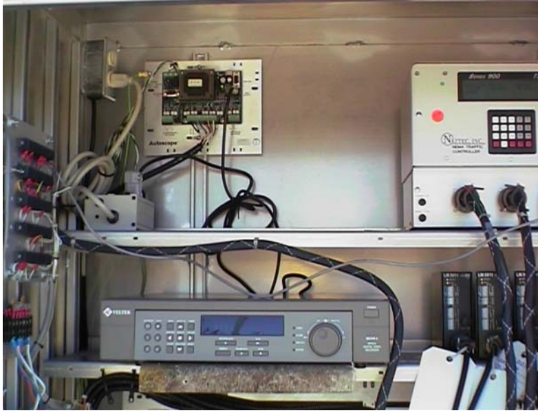
Photograph 2 Traffic Cabinet with Data Acquisition System and DVR
